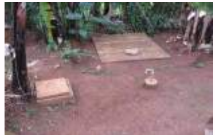
Un protected Main Gas Valve
