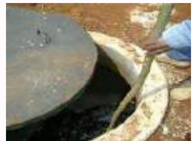
Expansion Chamber interior
