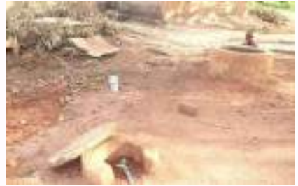
Protected Main Gas Valve
